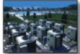
Twelve Heat Siphons Installed on Cranberry Twp., PA Community Pool
