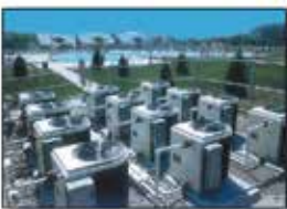
Twelve Heat Siphons installed on Cranberry Twp, PA Community Pool
